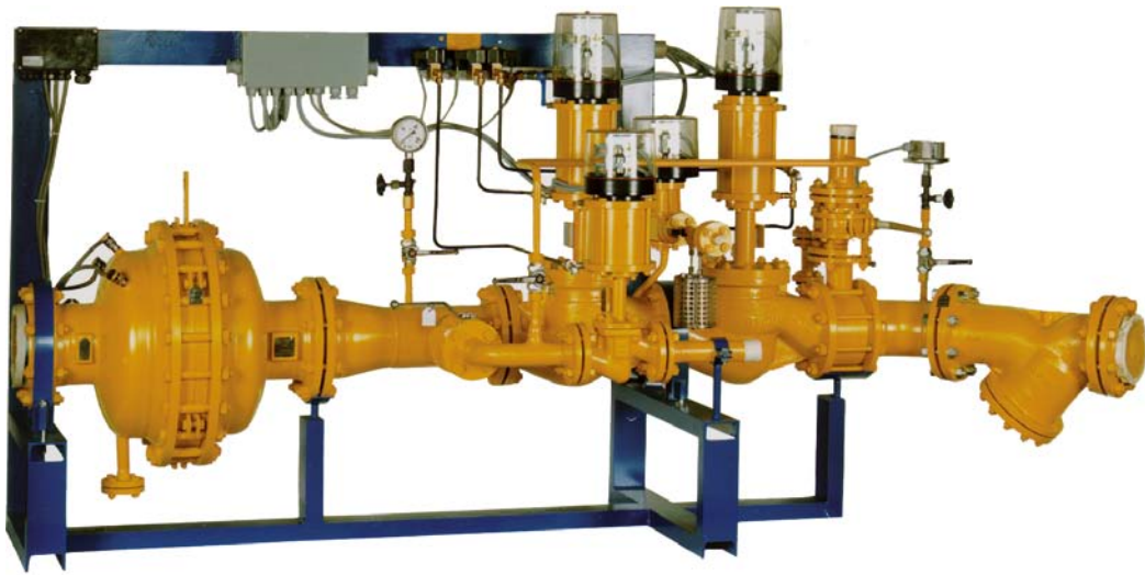
Fig. 9: Valve station for gas firing
