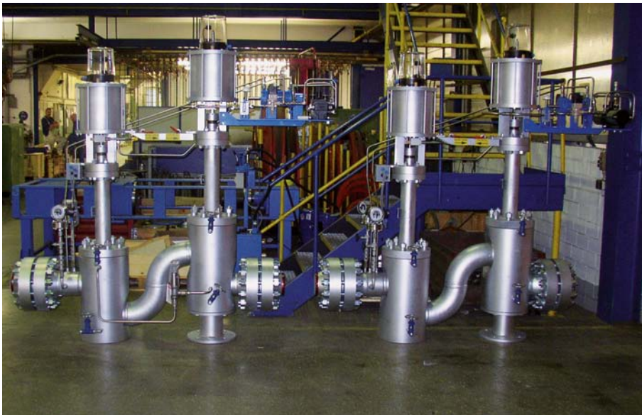
Fig. 6: Safety shut-off devices for thermal oil
